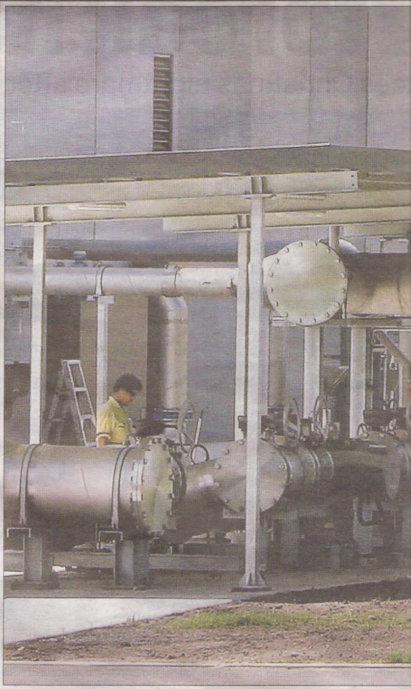
Pimpama Treatment Plant workers drank contaminated water for weeks
